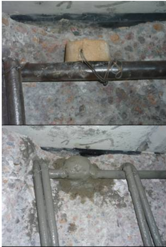
Figure 3. Galvanic anode type B installation procedure, (left) anode tied to the reinforcement as close as practically possible to the edge of the repair and (right) galvanic anode encapsulated in proprietary embedment mortar.
