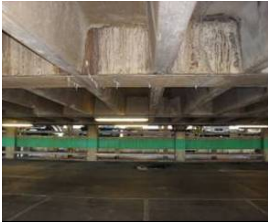
Figure 1. General condition of the MSCP's soffit indicating leaching, dynamic cracking and deterioration of the concrete elements.
